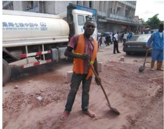
A labourer working on the rebuilding of Kinshasa’s main road, Boulevard du 30 juin , one of the first infrastructure projects under the Congo-China deal. From the information publicly available about the deal, it is unclear exactly how much infrastructure will be built and at what cost.
